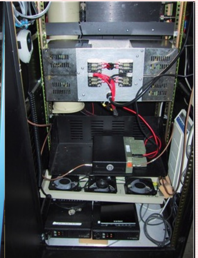
McKinney, Tx 145.350 VHF Repeater
